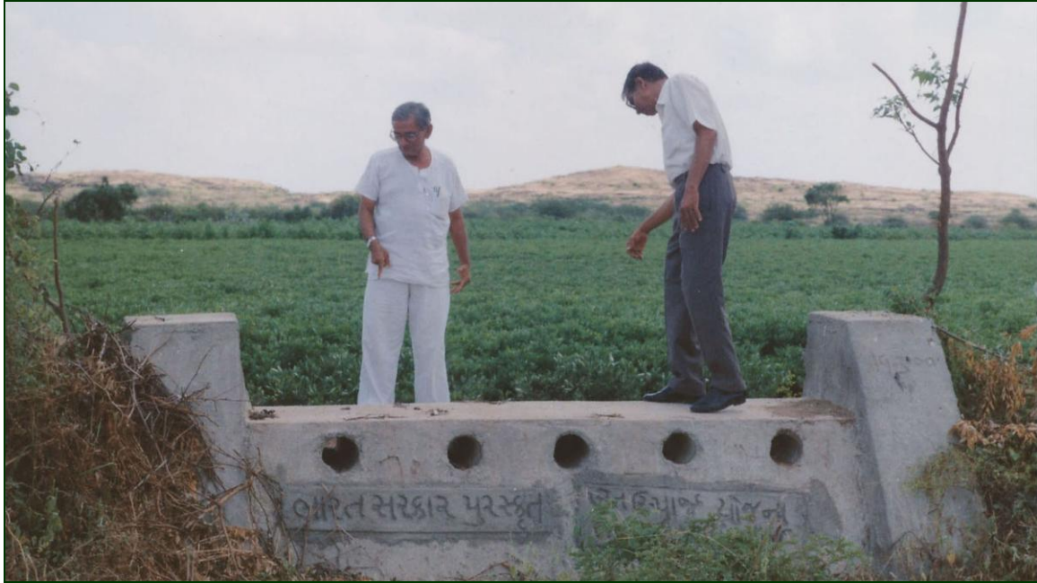
Fig. 41: Waste weir of a farm (farm outlet)
